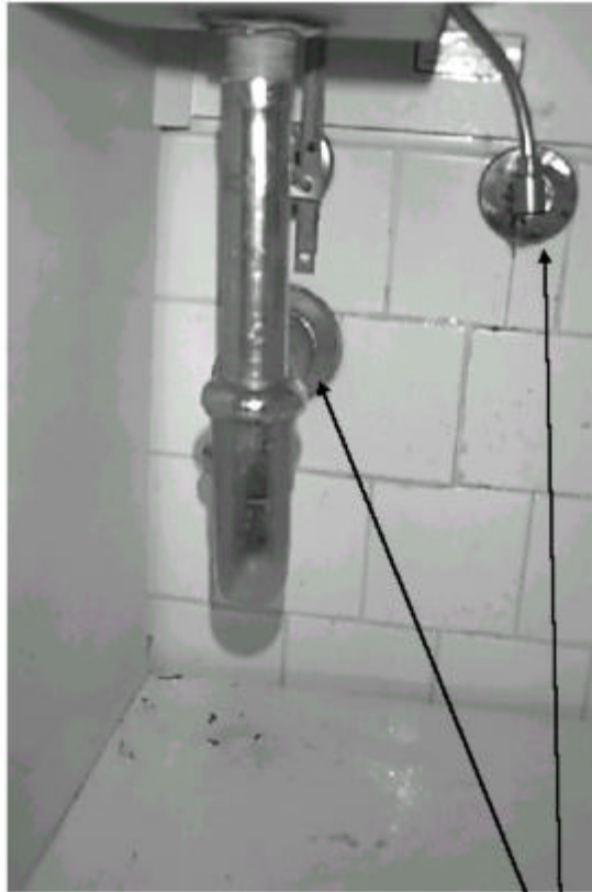
No gaps between pipes and wall
