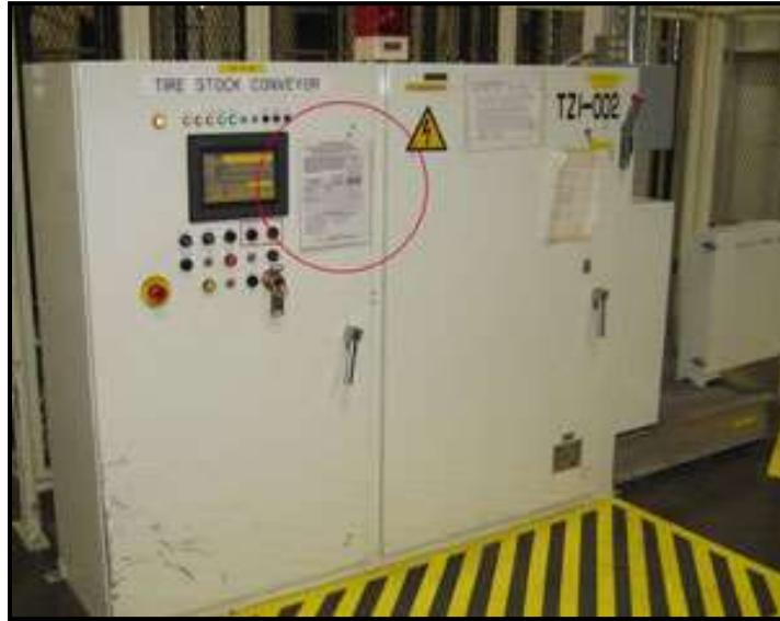
Equipment-Specific Energy Isolation Procedure shown in file on front of Equipment Control Panel.
