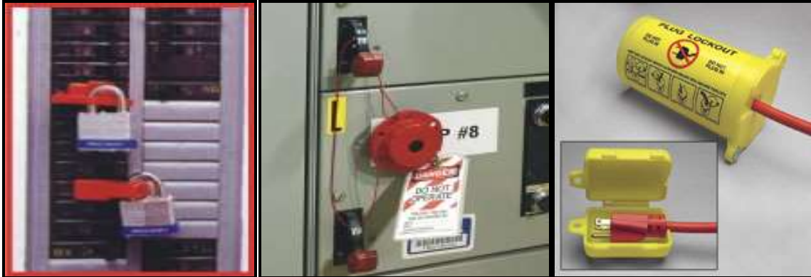
Locks and Tags on Single and Multiple Electrical Breakers
