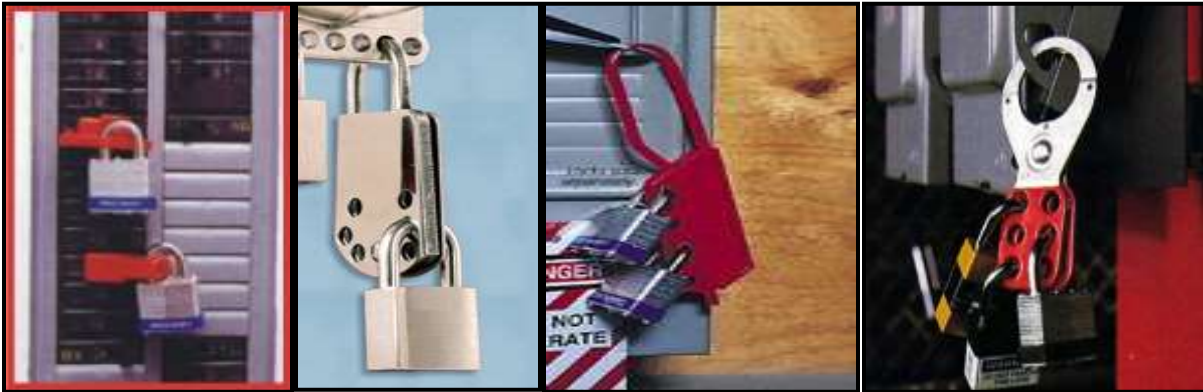
Electrical Panels shown “Locked Out”
