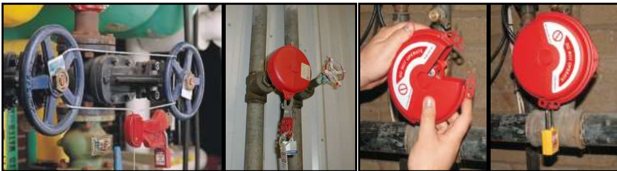
Piping shown “Locked Out”
